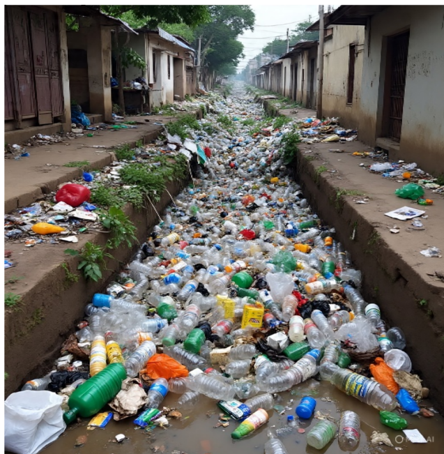
Figure 3. Drainage channel (Gutter) littered with solid waste. Source: Researchers' observation fieldwork
