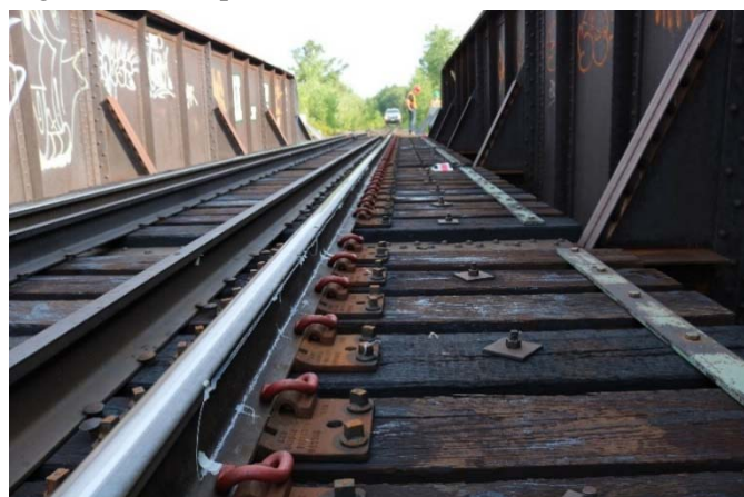
Figure 3 Fibre optic sensors on rail
