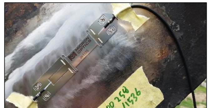
Figure 4 DFOS sensor mounted at the bottom chord of the old steel bridge and the FBG sensor SG7 is mounted very close to it at 14m from Abutment A, in order to
