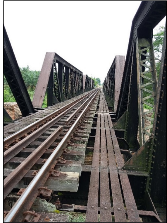
Figure 10 The connection and jointing system at the inner truss is more complicated than outer truss
