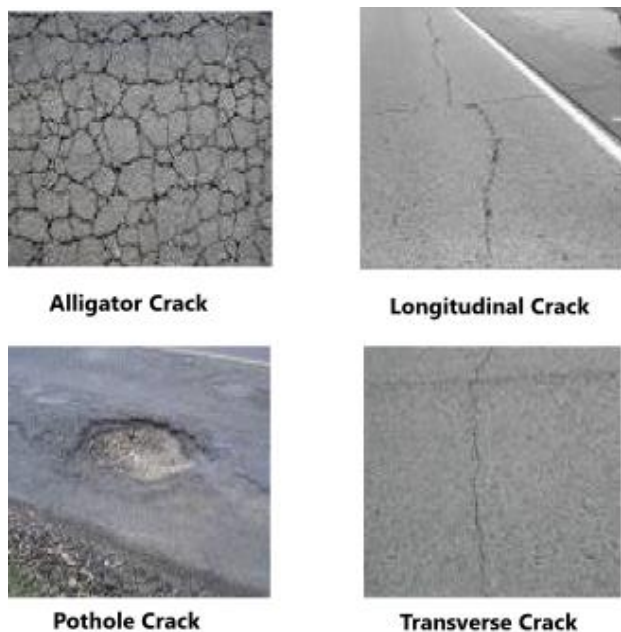
Figure 2 Examples of asphalt pavement crack.
