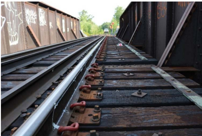
Figure 3 Fibre optic sensors on rail
