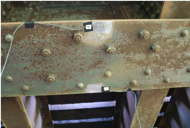
Figure 5 Strain gauges on the floor beam's bottom flange
