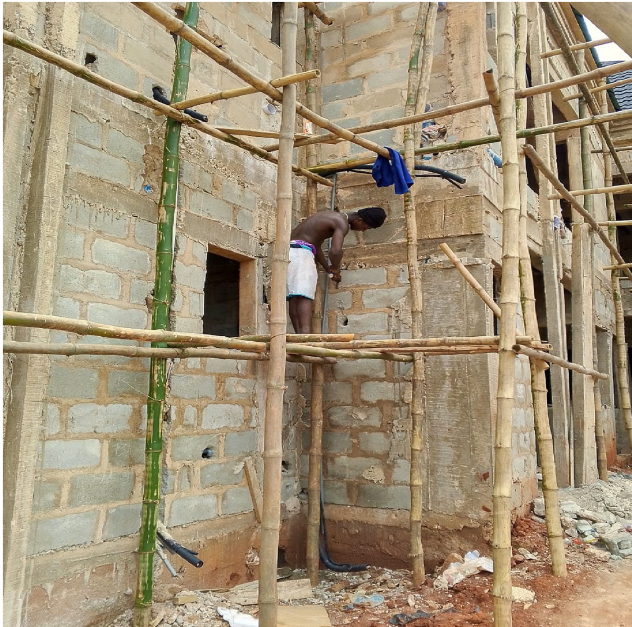
Figure 2. Carpenter fixing formwork without PPE. Site B (Source: Authors' work)
