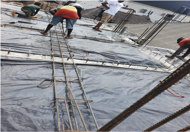
Figure 6. Iron bender and trainee on site tying beam reinforcement and stirrups without PPE. Site F (Source: Authors' work)
