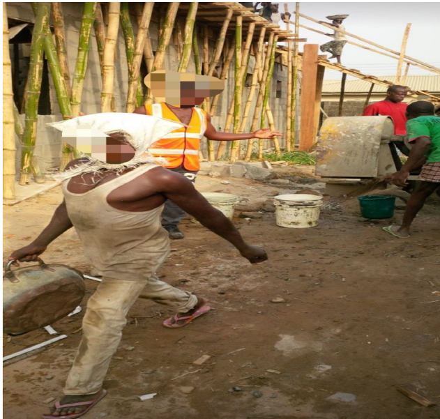
Figure 1. Artisans loading the concrete mixer without PPE. Site A (Source: Authors’ work)
