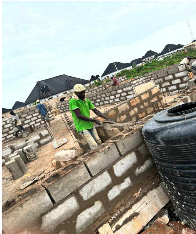
Figure 4. A block layer applying mortar without PPE kits. Site D (Source: Authors' work)
