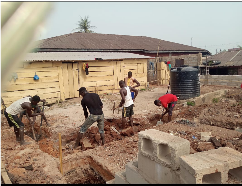
Figure 7. Excavators, excavating foundation trenches without PPE. Site G (Source: Authors' work)
