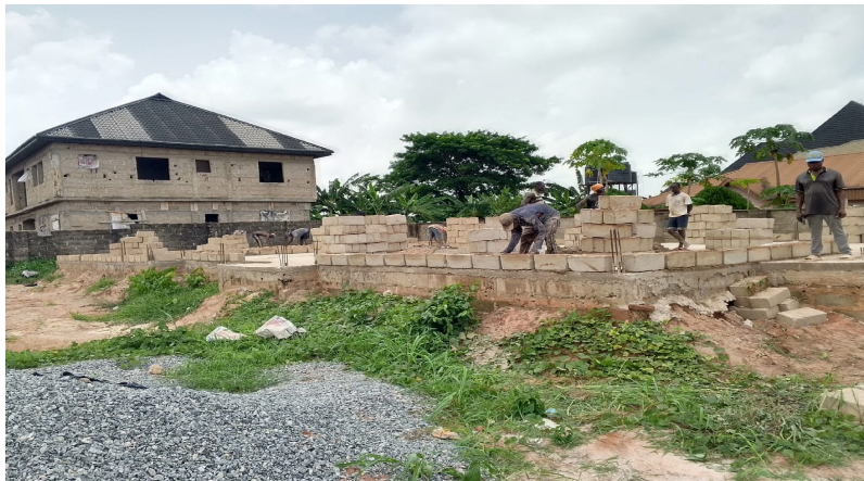
Figure 5. Block layers and helpers on site laying blocks without PPE. Site E (Source: Authors' work)
