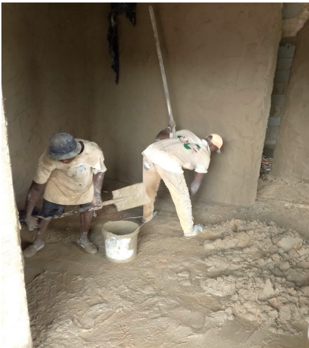
Figure 3. Mason and helper rendering the wall without PPE. Site C (Source: Authors' work)
