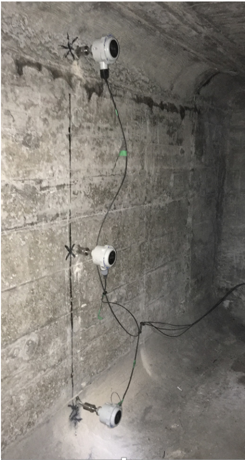
Figure 7. Photograph of installed temperature sensors (photo: WSP)
