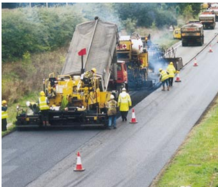
Repairing local transport infrastructure is vital to improving the nation's transport system
