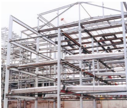
Cross-section classification, laterally unrestrained beams, prying action in bolted connections and portal frame stability are the subject of significant safety-related, technical up-dating in the new BS 5950: Part 1
