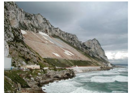
Gibraltar rainfall catchments were in use and well maintained until at least 1987
