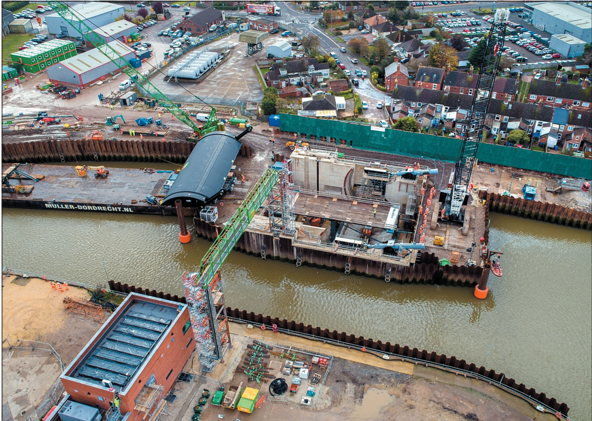
Figure 7. Integration of permanent and temporary works in the cofferdam enabled the gate to be driven into position from a barge using a self-propelled modular transporter (Environment Agency)
