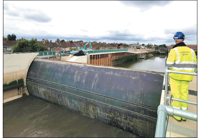
Figure 4. The 362 t rising sector gate is 26 m wide, 11 m high and became operational at the end of 2020 (Environment Agency)
