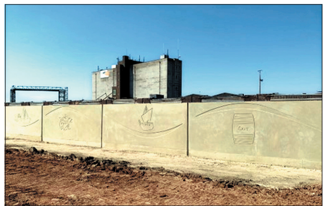
Figure 6. Murals on the new right bank floodwall reflect the town's maritime history and were developed in consultation with the local community (BAM Nuttall and Mott MacDonald joint venture)
