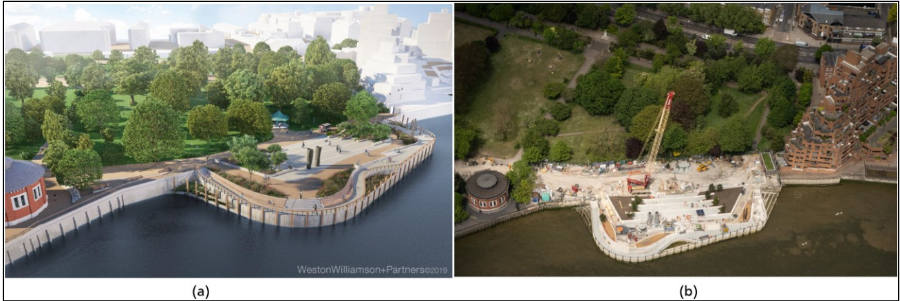
Figure 3. King Edward Memorial Park Foreshore: (a) 2013 visualisation (@Thames Water); (b) construction nearing completion in 2025 (photo credit: Patricia Rayner)
