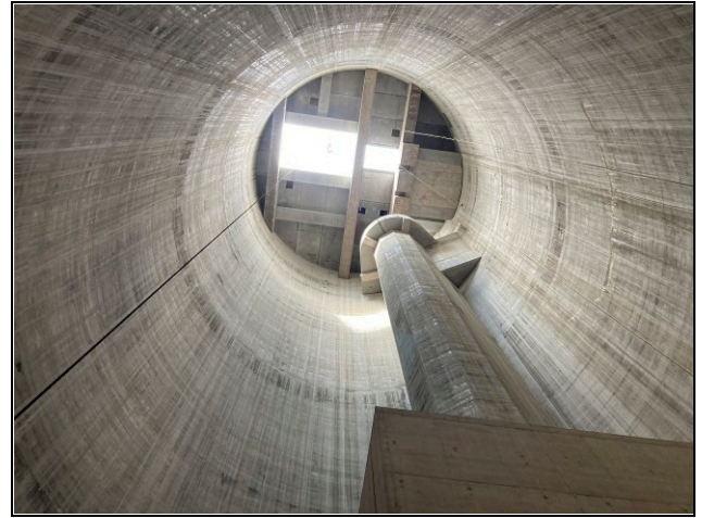
Figure 8. Drop shaft with completed secondary lining, lined vortex drop tube and roof slab
