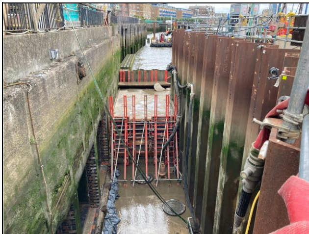
Figure 6. NESR diversion channel – construction of the final connection with the existing sewer
