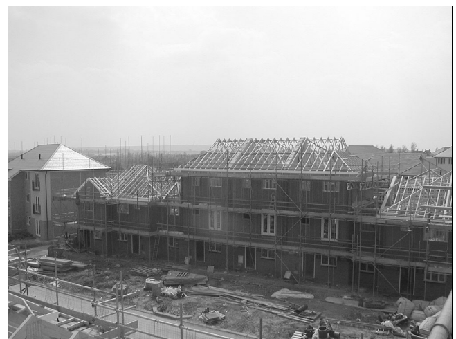
Fig. 2. Marlow's Timber Engineering has achieved comprehensive chain of custody certification with BM TRADA
