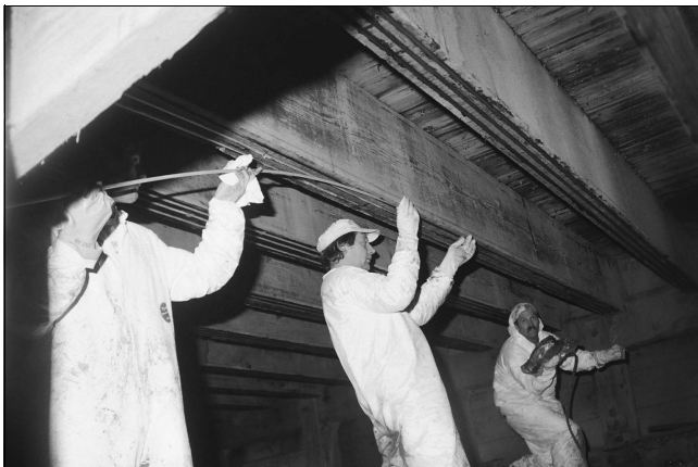
Fig. 5. Reinforcement of Tourand Creek Bridge, Canada. Rotaflex rods are being pressed into slots filled with Rotafix CB10T SS adhesive, © Rotafix Ltd
