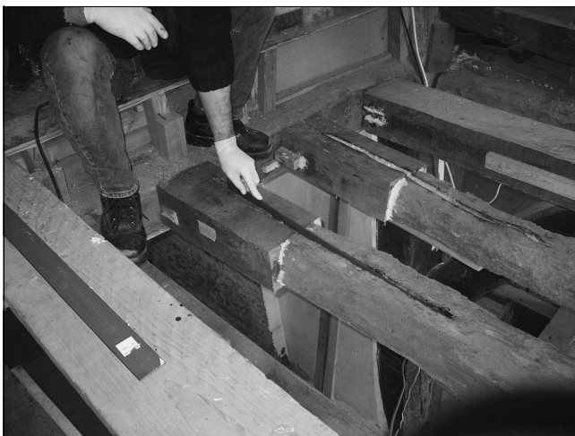
Fig. 6. CFRP plates being dry-fitted into slots before adhesive installation. The original beams are to the right and the new sections to the left, © Rotafix Ltd
