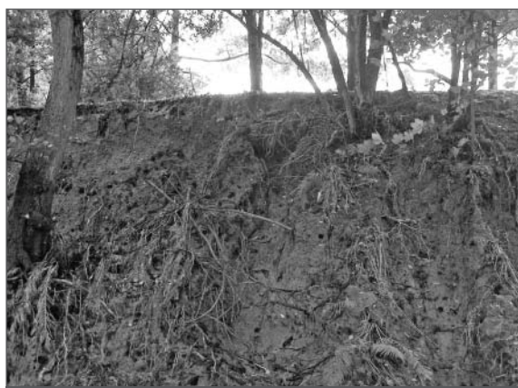
Figure 1. Eroded downstream shoulder
