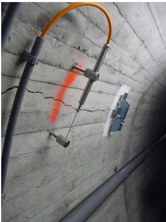
Figure 17. Cracking to gallery
