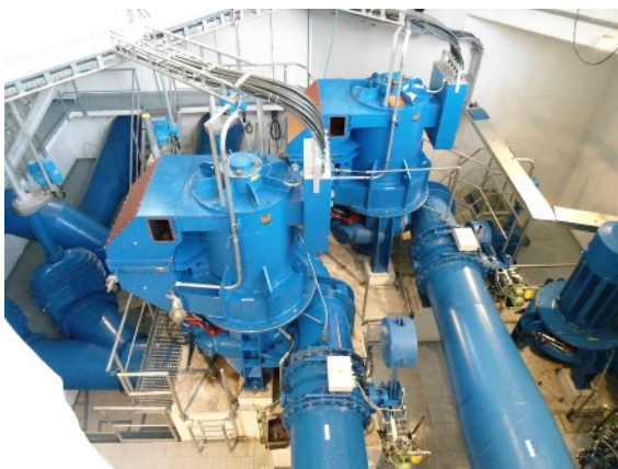
Figure 8. Compact power station with Francis turbines
