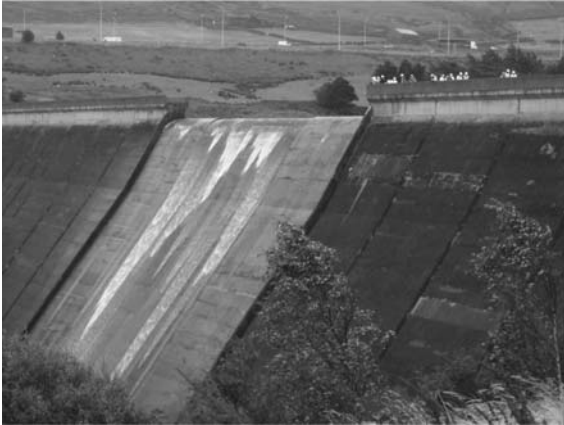
Figure 2. Boothwood dam with M62 in background and BDS conference members on dam
