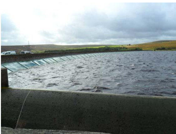
Figure 1. Geomembrane on upstream face of Winscar dam
