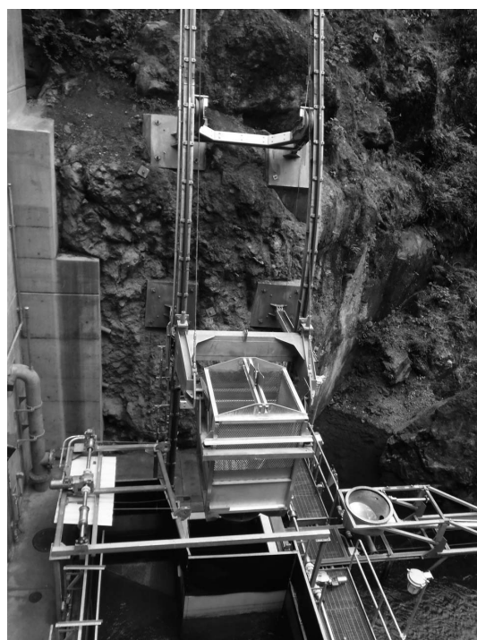
Figure 5. Fish collection system at Cushman dam no. 2
