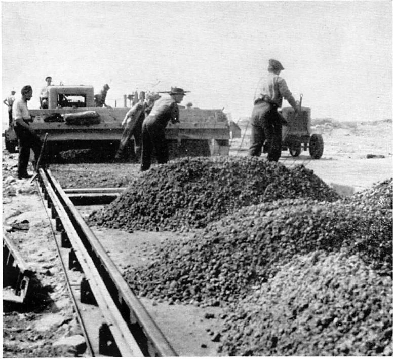
CONCRETE DUMPED ON FORMATION IN FRONT OF BLADE SPREADER. ON THE LEFT ARE RAILS, TO CARRY SPREADING AND COMPACTING PLANT, SECURED TO SIDE FORMS
