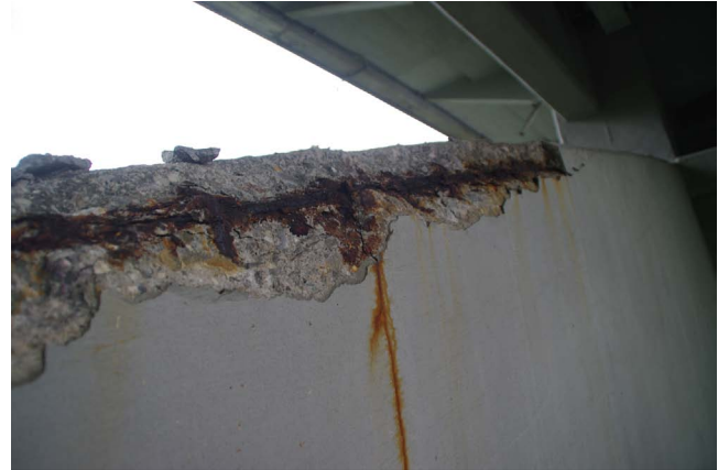
Figure 7. Example of damages to the arches
