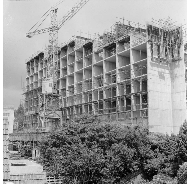
Figure 2. GWF under construction (14 November 1957). Source: Evening Post Collection, Alexander Turnbull Library, National Library, Wellington, NZ. Reference: EP/1957/4364-1-F
