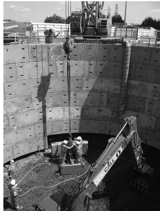
Figure 8. Erection of pre-cast segments for National Grid's LPT project (NG, 2015). The ground is exposed prior to erecting the shaft lining (EBS construction)
