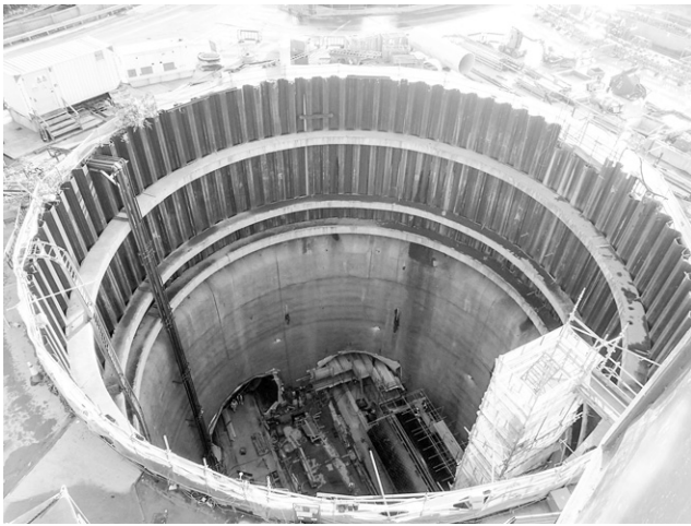
Figure 10. A 28 m dia. and 39 m deep TBM launch shaft at Limmo Peninsula comprising pre-installed sheet piles (SBE construction) and a SCL (EBS construction)
