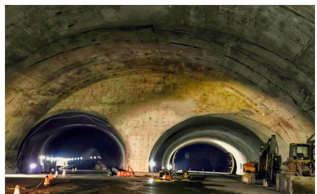
Figure 1. Maximum section of the Liantang tunnel in China (taken from Tan et al. (2021))
