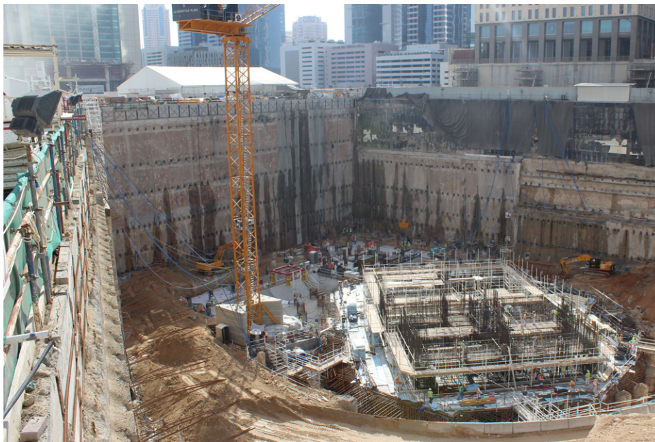
Figure 2. South end of excavation at its greatest extent for the ICD Brookfield Place development in Dubai (taken from Smith et al. (2021))
