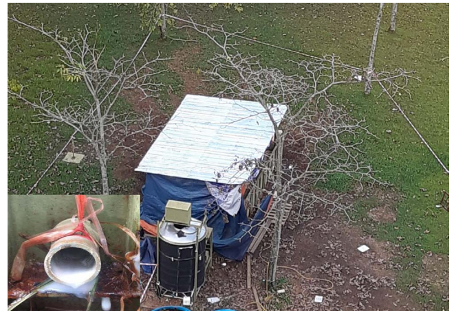
Figure 7. Leakage of ammonium-rich effluent in a 10 m 3 sandbox during an outdoor bio-cementation treatment
