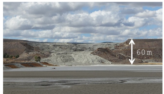
Figure 3. NTSF slump viewed from Southern Tailings Storage Facility embankment
