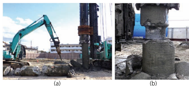
Figure 2. Existing pile that broke in the process of removing it: (a) full view of removal work; (b) state of broken existing pile
