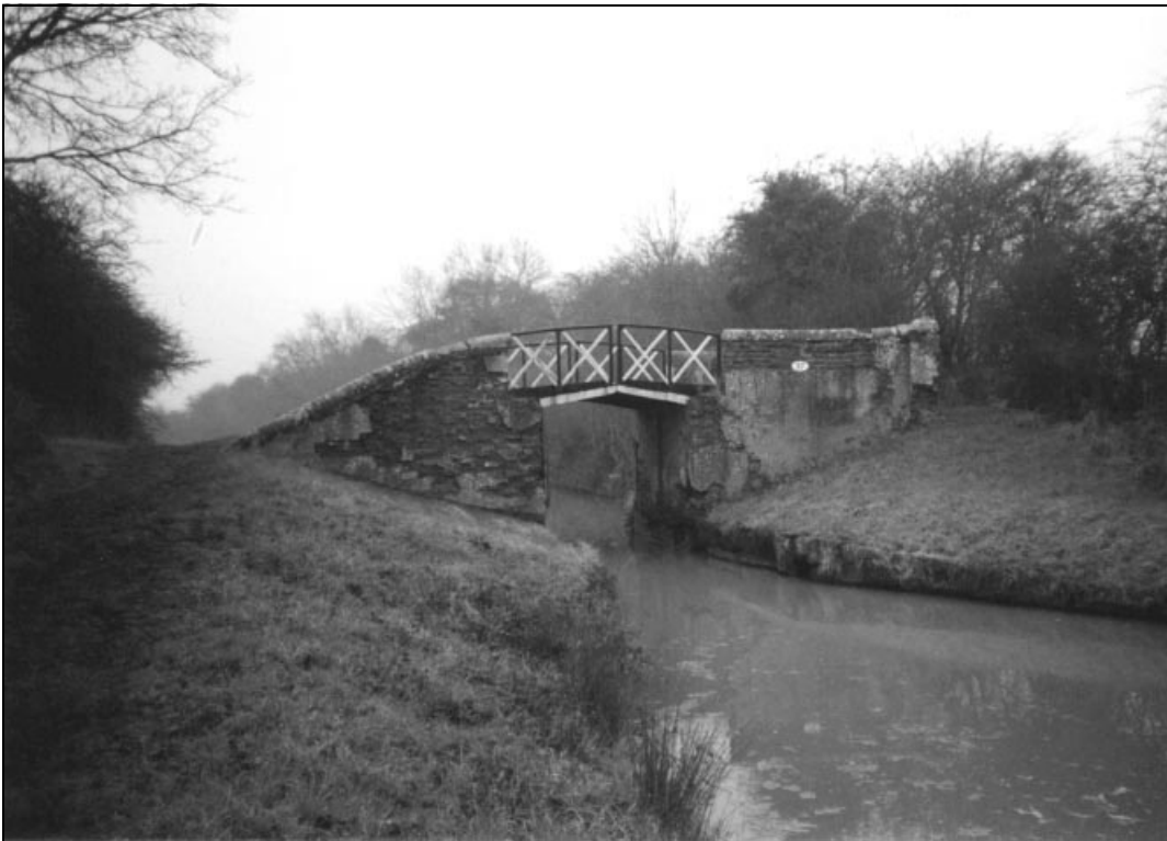
Fig. 3. Packhorse bridge—long-term damage and unsympathetic repair
