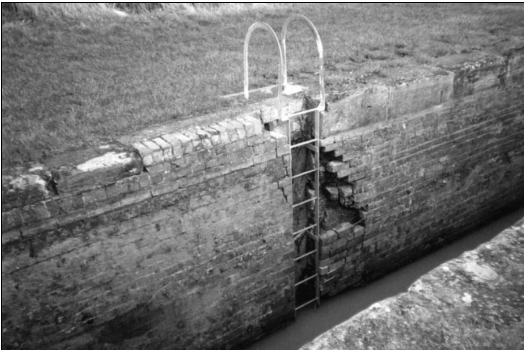
Fig. 6. Failure of unbonded facing skin to lock
