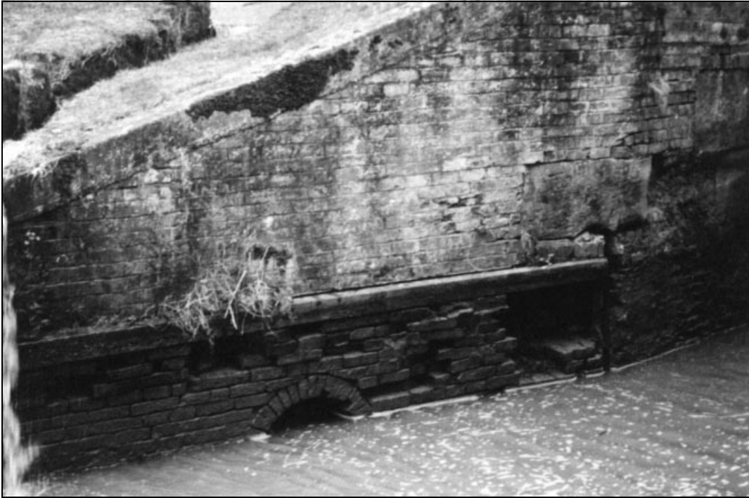
Fig. 7. Severe damage above and below water line (lock 50)
