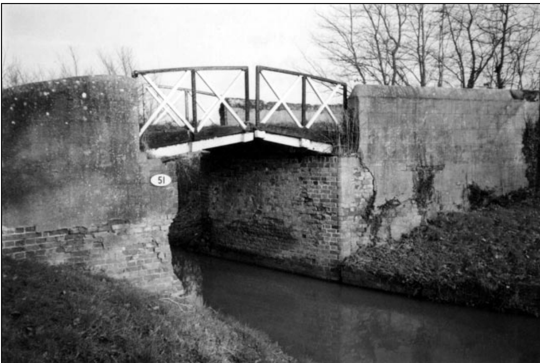
Fig. 4. Packhorse bridge—long-term damage and unsympathetic repair
