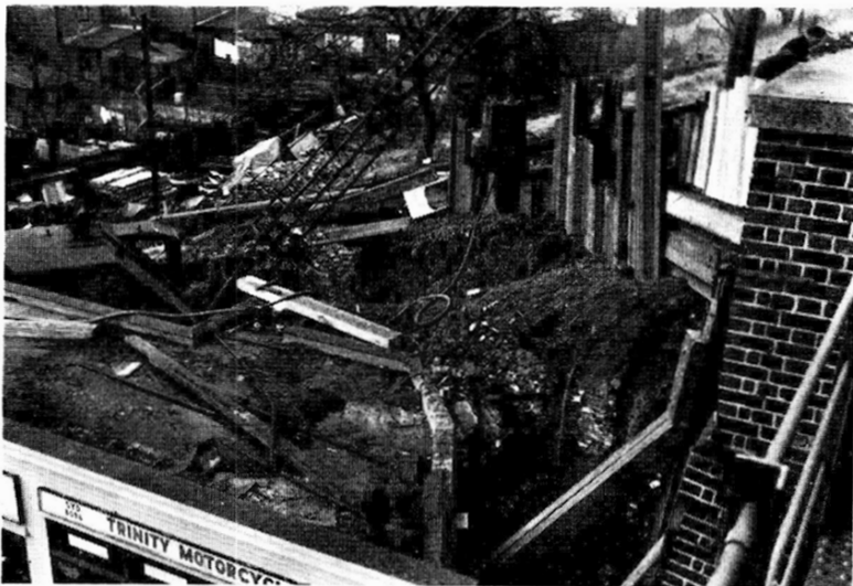
FIG. 50: EMERGENCY MEASURES TAKEN DURING SUNDAY TO OPEN LINE TO TRAFFIC AFTER COLLAPSE OF CIRCULAR WING WALL
