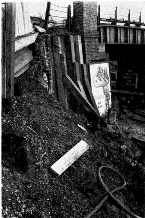
FIG. 49: COLLAPSE OF CIRCULAR WING WALL CAUSED BY EARTH PRESSURE DUE TO SLIP
