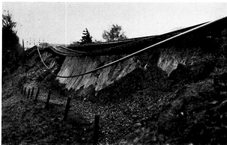
FIG. 61: SLIP AT HOOK, SOUTHERN REGION 27 DECEMBER 1960. FIRST STAGE—UP LOCAL UNDERMINED
