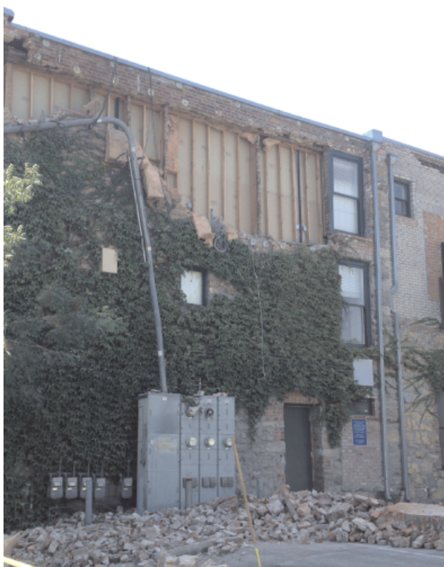
Figure 1. This brick-and-timber building sustained significant damage despite the out-of-plane anchors seen along the top of the wall. Copyright Arup (2014)
