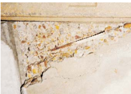
Figure 6. Photograph of observed damage
