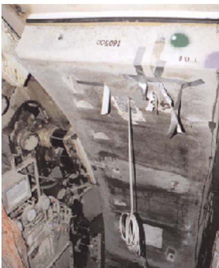
Figure 11. Installation of an instrumented segment at the Botlek Railway Tunnel to measure assembling stresses
