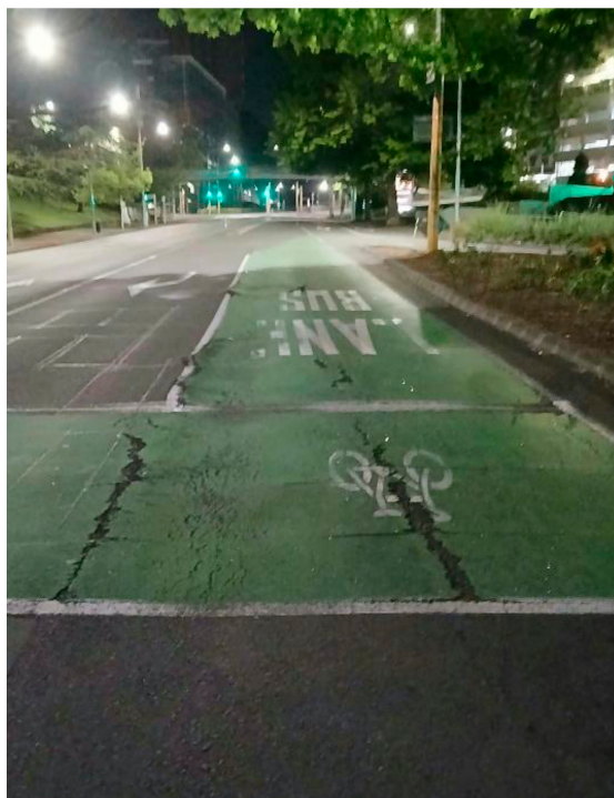
Plate 8. Progressive views of surface damage and low-lighting under mature trees. These micro-level hazards undermine Auckland Transport’s luminance standards and rider safety
