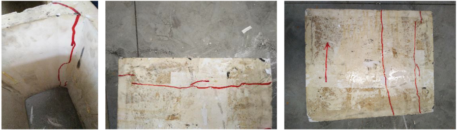
Cracked segment of lining structure (11#)
