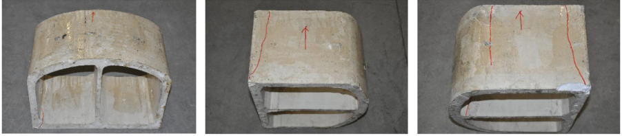
Cracked segment of lining structure (7# ~ 8#)
