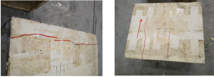
Cracked segment of lining structure (7#) (a)
