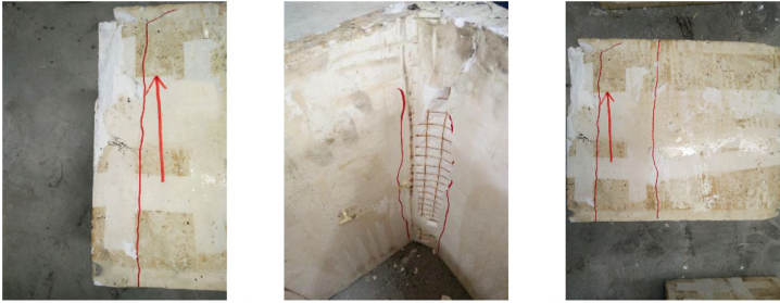
Cracked segment of lining structure (8#) (b)
