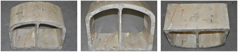
Cross-fault cracked section of lining structure (9#)
