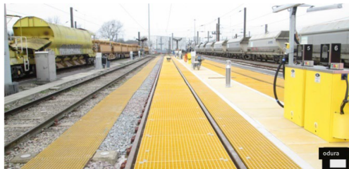
Composite grating walkways between railway lines
