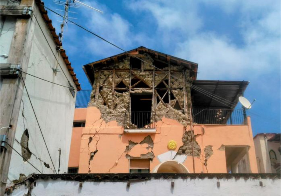
Figure 9. Barrack house – Shack house in Casamicciola after the 2017 earthquake Source: Photo by Giovanni Gugg – May 24th, 2018. (Gugg, 2024)
